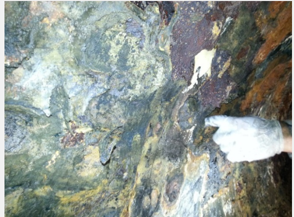
Subject Wastewater Line: The deteriorated pipe section post-cleaning and pre-lining. Evident is significant wall loss and major perforations from aggressive H 2 S erosion.
