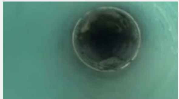
Installed PipeArmor: Shown in foreground is the completed PipeArmor® polymer pipe-in-pipe. In background, for contrast is the downstream section which remains in service in its original state.
