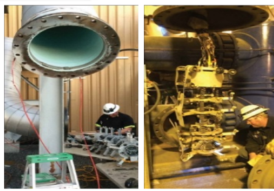
Robotic versatility – Left: Completed 45 deg. mitre into unit. Right: SD1 robot makes insertion for vertical lining segment.
