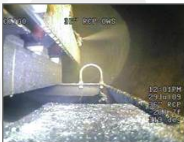
Process Step: The robotic grouting process is shown, with the application of the acrylamide to seal and fill exterior voids.
