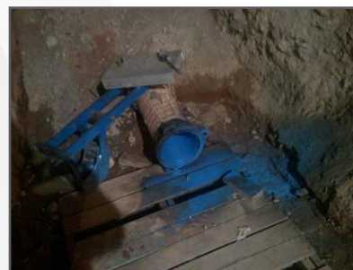
Post Lining: The buried pipe (under major improvements) is shown with its blue liner which protects against erosion from abrasion and corrosion.
