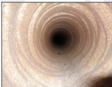
Process Step: The pipe walls were thoroughly cleaned of corrosion and profiled to receive the liner. Note perforations at bottom of pipe radius.
